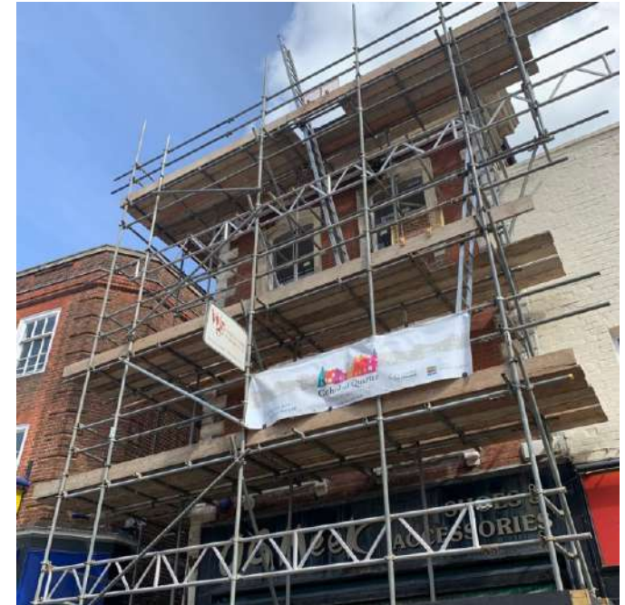
Works at 14 Westgate Street as part of the Cathedral Quarter HSHAZ. Photo: GCC.
