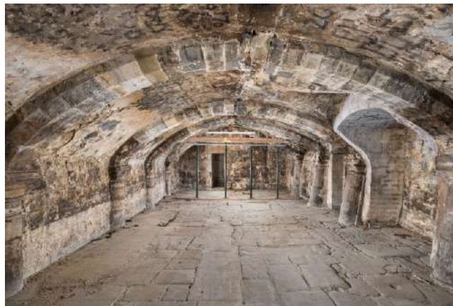
The twelfth-century undercroft in the Grade I listed Fleece Hotel. Photo: Historic England Archive.
